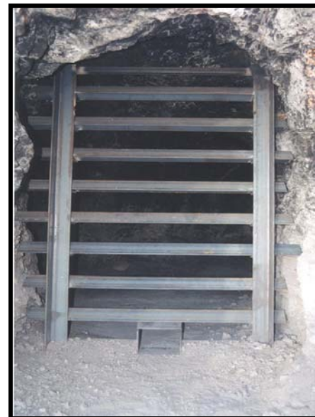
Bat gate installed at Copper Mountain Mine
