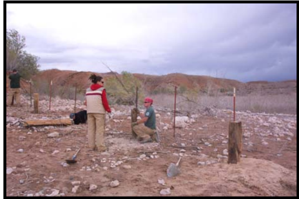
Nevada Conservation Corps members install post and cable barriers near the terminus of Lake Mead's Approved Road 111 in the Overton Arm.
